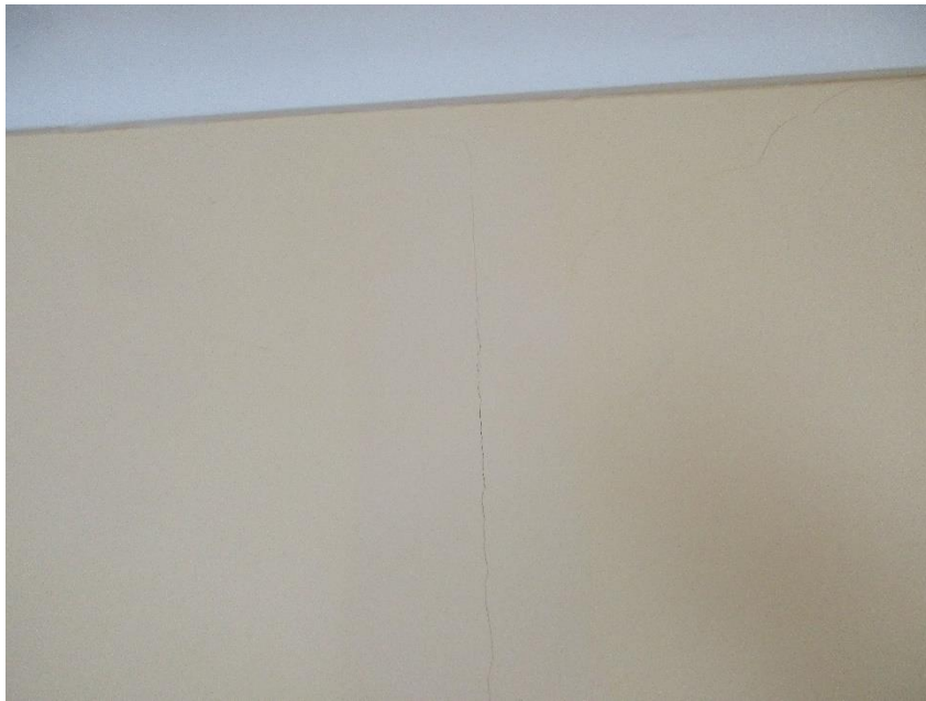
60 Interior – Lounge – Cracking to wall – joint between plasterboard and solid masonry to filled opening to dining room.
