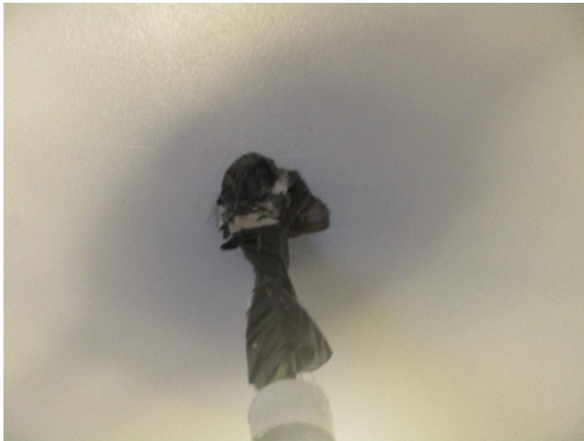
68 Interior – Landing – Bare wires to pendant – fitting is hanging and not secured – replacement required.
