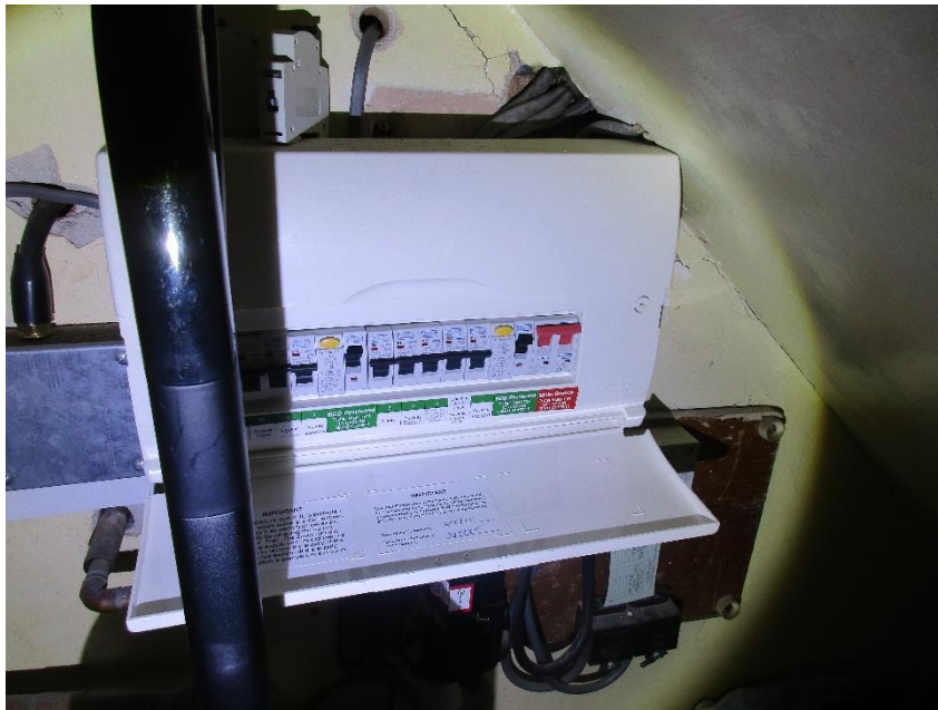
56 Interior – Entrance hallway – Under stair cupboard – consumer unit.
