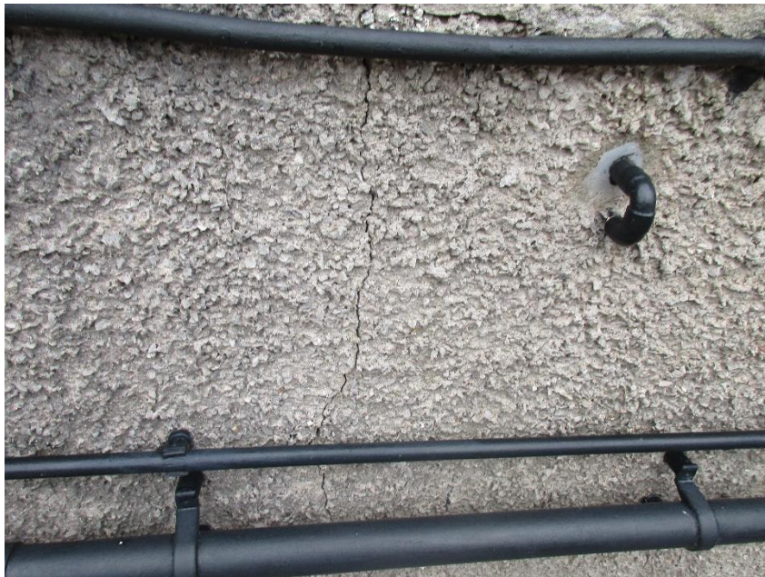
22 Exterior – Cracking and hollow render noted – repairs will be required.
