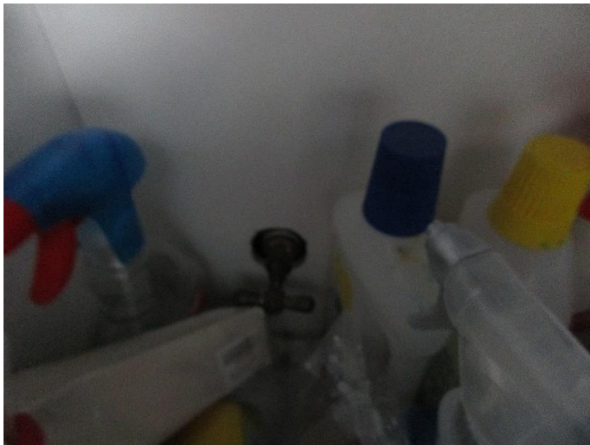
66 Interior – Kitchen – Mains water stop tap – unable to see supply pipe.
