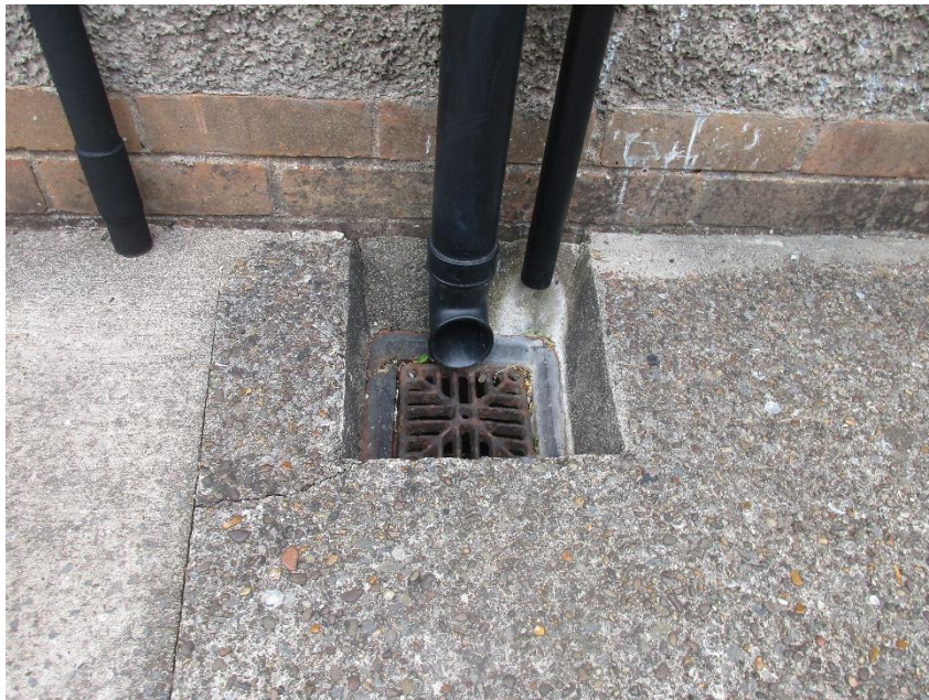
28 Exterior – Drains will require periodic clearing.
