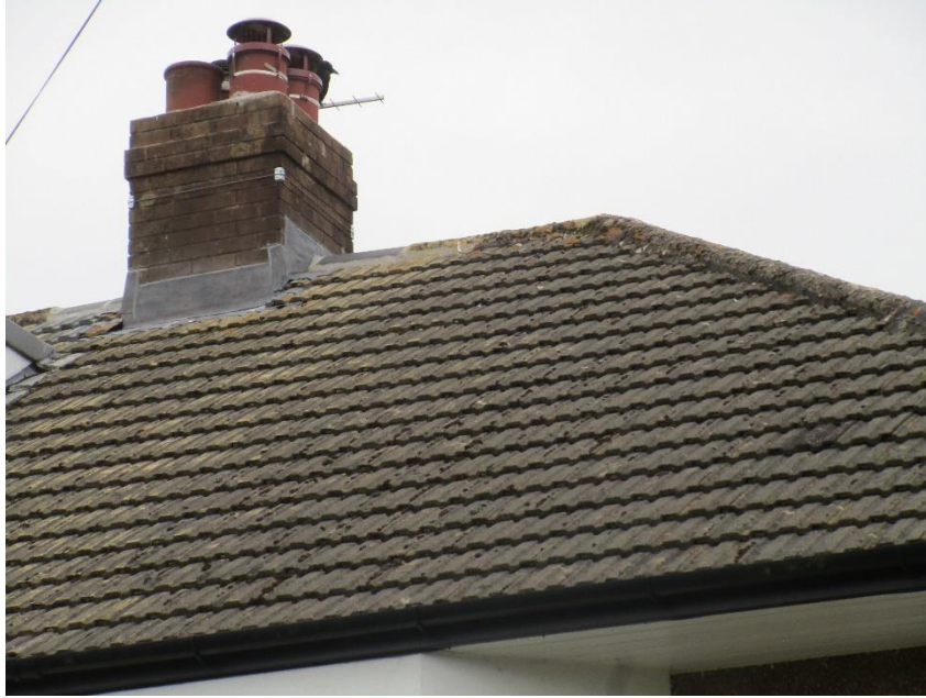
05 Exterior – Concrete interlocking tile roof covering – moss and lichen growth noted – not excessive.
