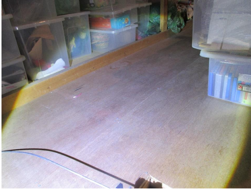
13 Interior – Roof Void – Boarding over blanket insulation will reduce its efficiency.
