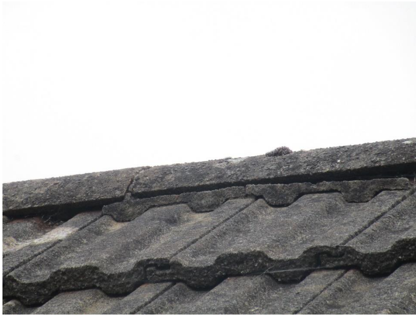
46 Exterior – Garage – Cracked and missing cement bedding mortar to ridge tile.
