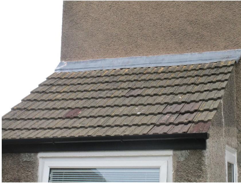
09 Exterior – Rear extension roof covering – replacement tiles noted – weatherproofed to rear wall in lead.
