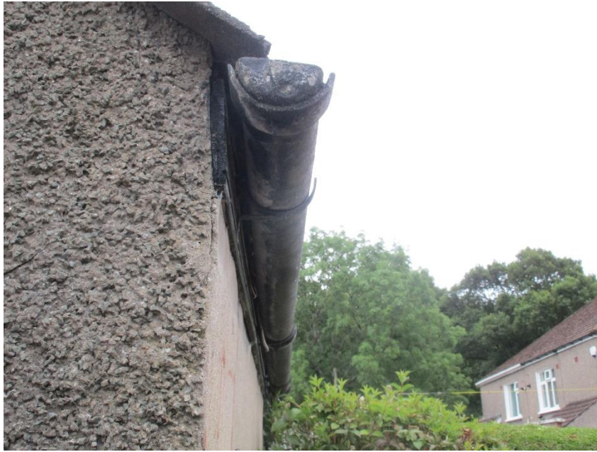
47 Exterior – Garage – Metal gutter to right side – limited inspection – cannot rule out asbestos.
