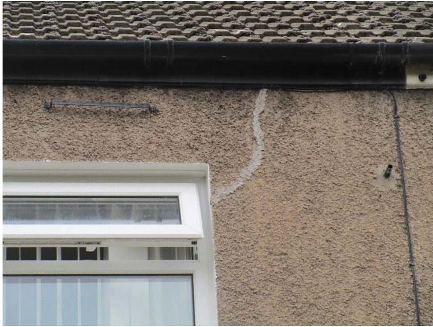
23 Exterior – Repairs to cracks to rear elevation – poorly finished.
