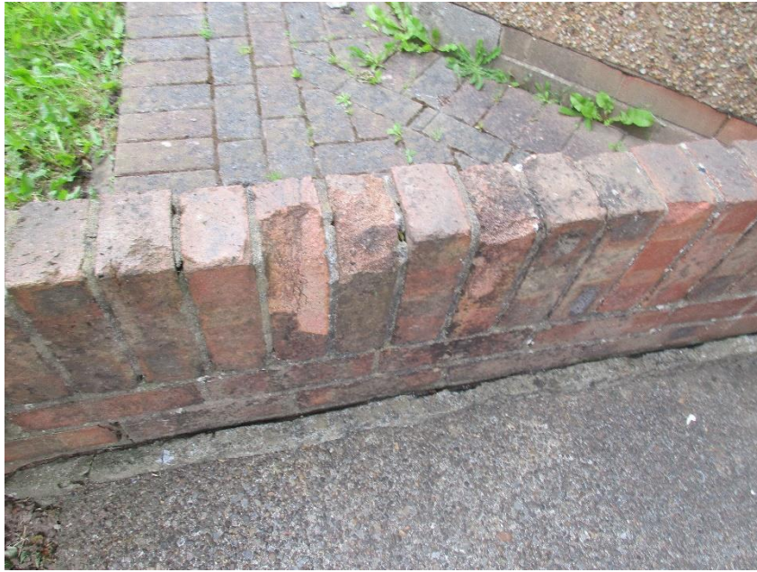
33 Exterior – Front left boundary – damage noted to bricks.
