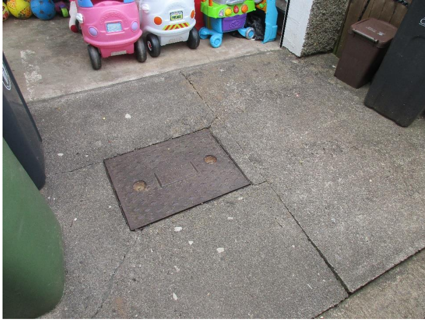
39 Exterior – Frontage – cracking and unevenness to concrete driveway and pathways.
