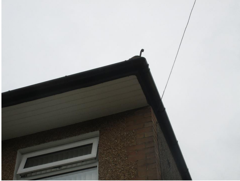
27 Exterior – Timber fascias and soffits will require periodic re-decoration.
