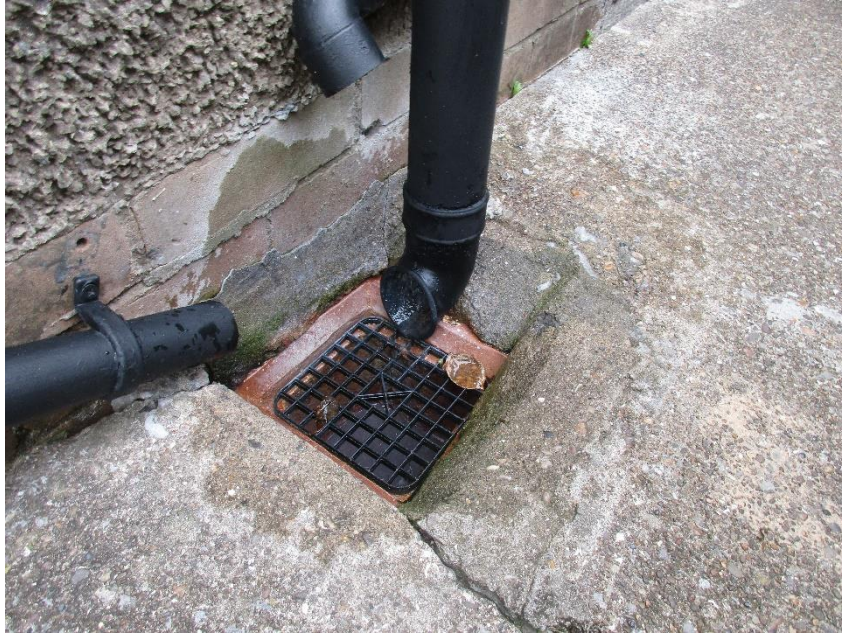
29 Exterior – Drains will require periodic clearing.
