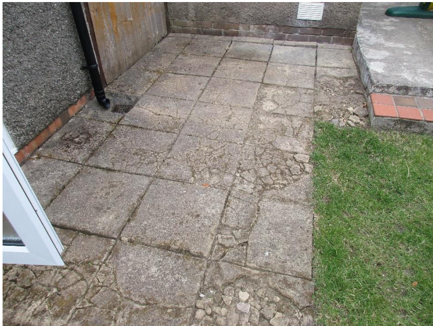
44 Exterior – Cracking, damaged and uneven patio slabs.
