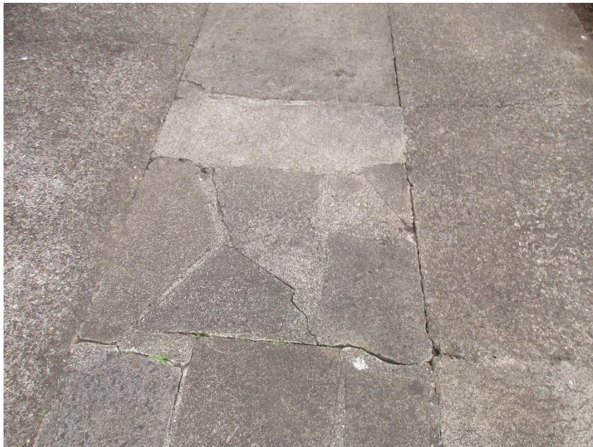
38 Exterior – Frontage – cracking and unevenness to driveway and pathways.
