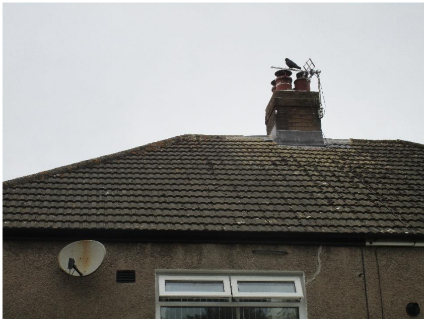
08 Exterior – Rear of Main roof – moss and lichen growth – not excessive.
