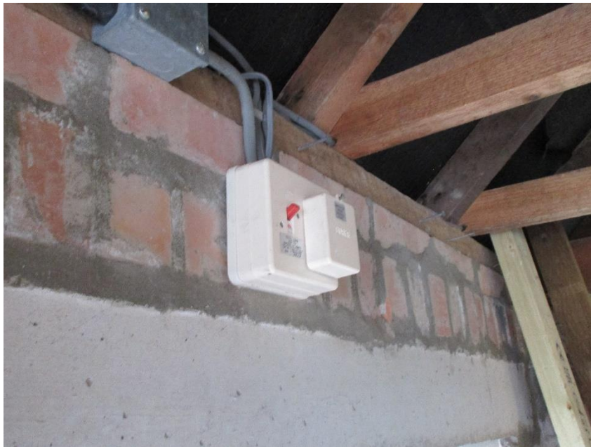
50 Interior – Garage – Wired consumer unit – periodic inspection required.
