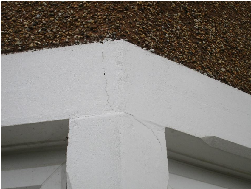
20 Exterior – Cracking to concrete to bay window – not excessive – periodic repairs and re-decoration will be required.
