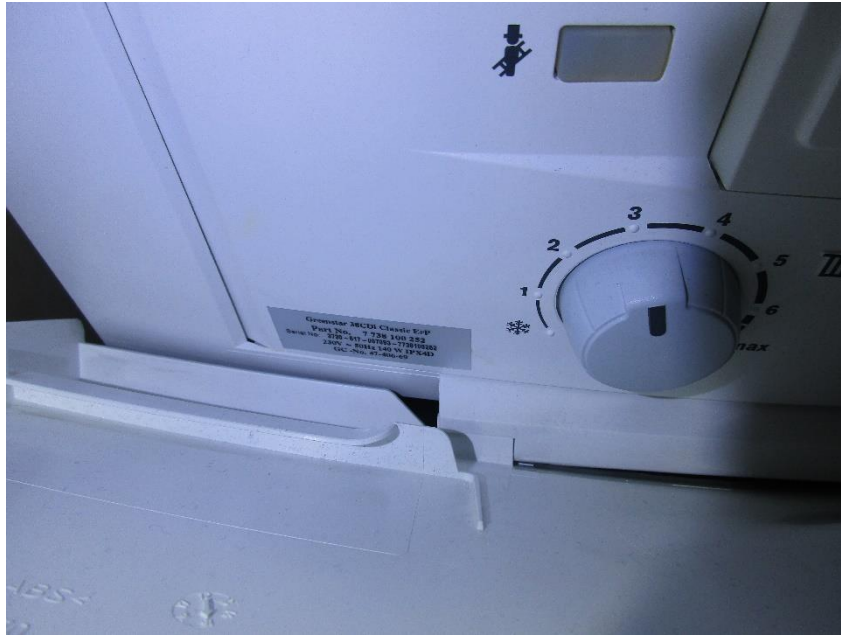
57 Interior – Entrance hallway – Understairs cupboard – Worcester condensing boiler.
