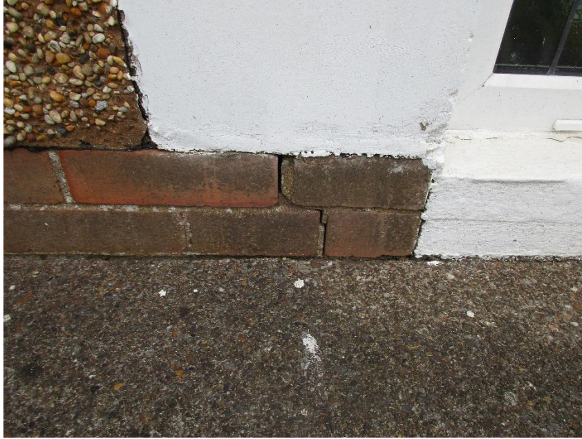
19 Exterior – Pointing repairs required to brickwork to low level – DPC visible.
