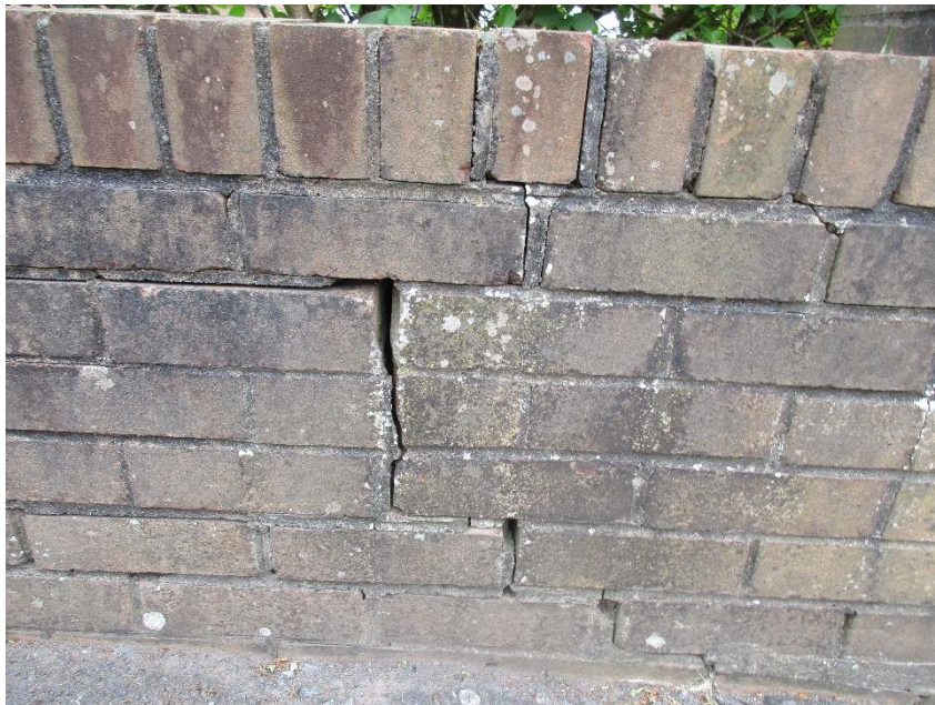
36 Exterior – Front Boundary – cracking to brickwork.
