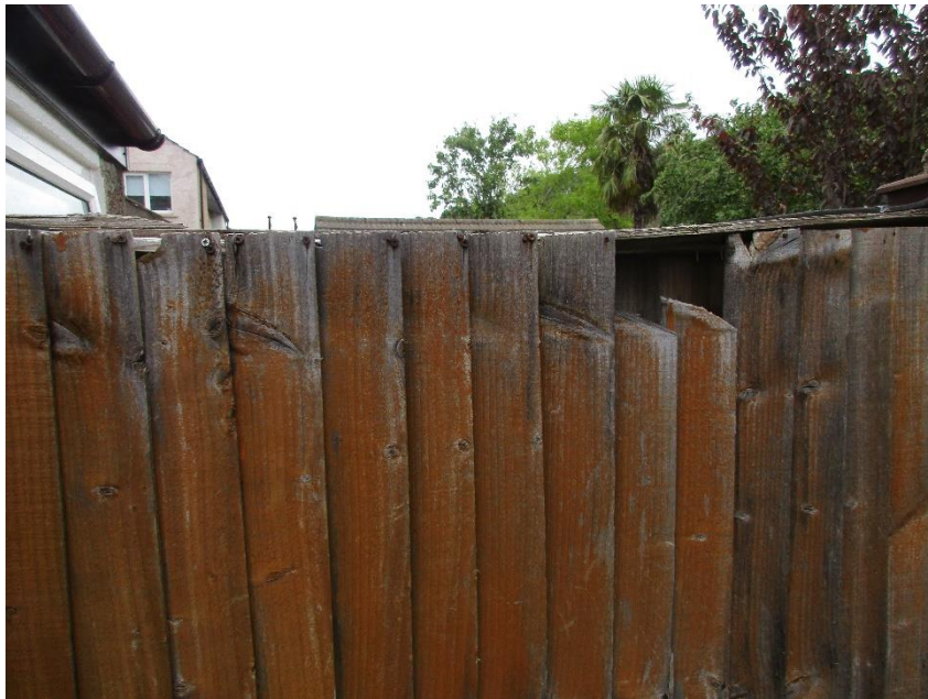
40 Exterior – Damage to timbers between driveway and rear garden.
