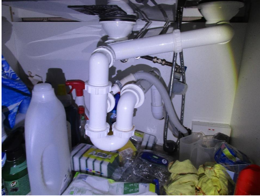
65 Interior – Kitchen – Plastic waste pipes and copper and flexible hose supply pipes.
