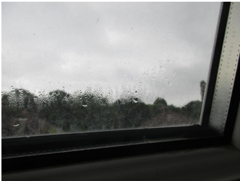
70 Interior – Bedroom One – Misting noted to glazing – seal has failed.
