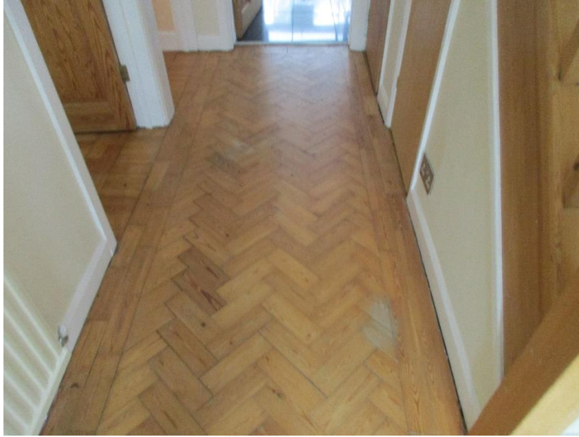
55 Interior – Entrance hallway – wear noted to parquet flooring.
