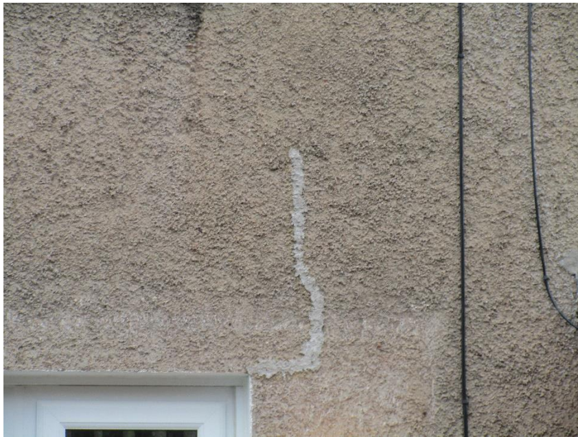
24 Exterior – Repairs to cracks to rear elevation – poorly finished.
