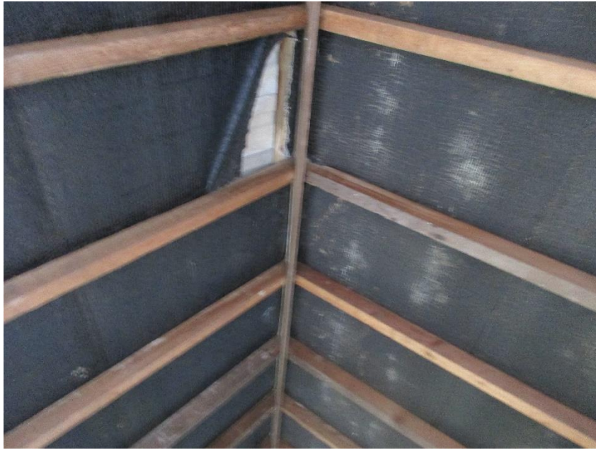
49 Interior – Garage – Tearing noted to under felting.
