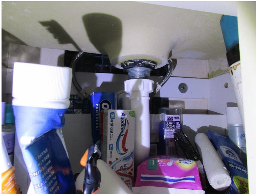
74 Interior – Bathroom – Plastic waste pipes and flexible hose supply pipes.
