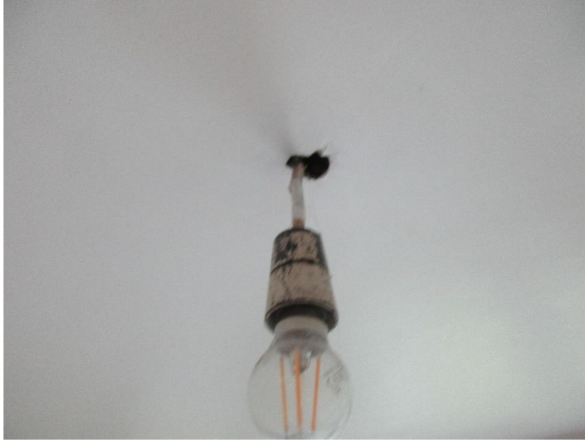
53 Interior – Entrance Hallway – Older style fitting – pendant not secured to ceiling.
