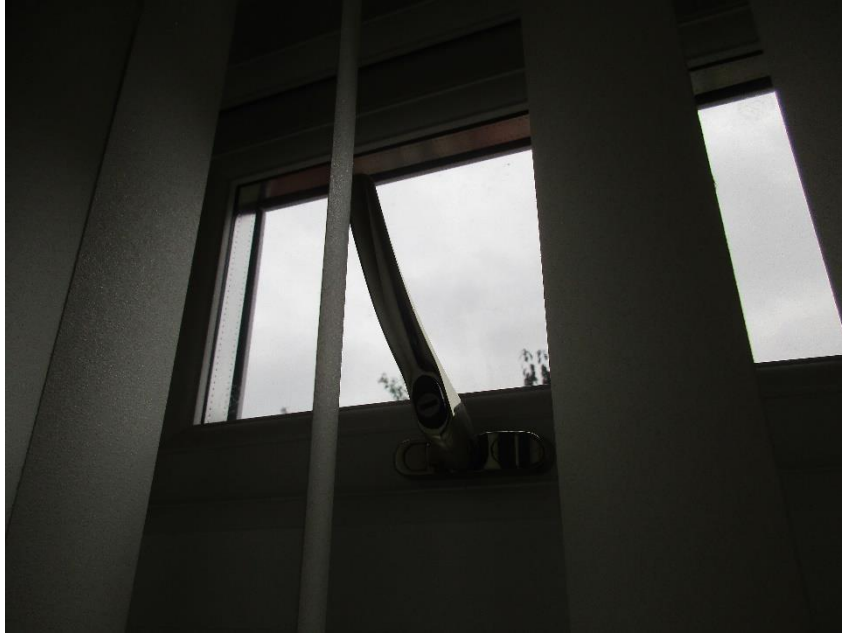
63 Interior – Dining Room – Top left window did not open even though handle turned.
