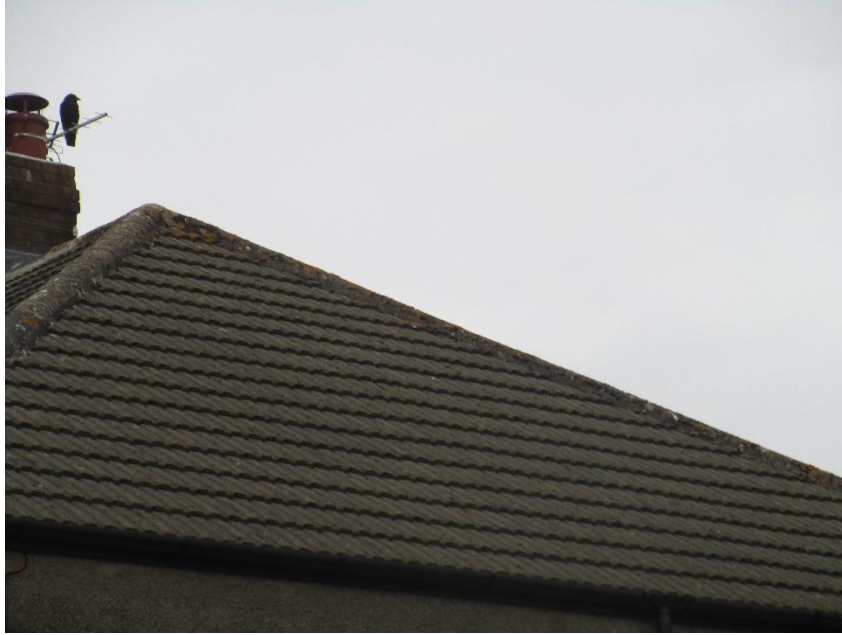
07 Exterior – Side of Main roof – moss and lichen growth – not excessive.
