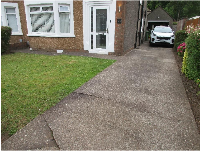
37 Exterior – Frontage – cracking and unevenness to concrete driveway and pathways.
