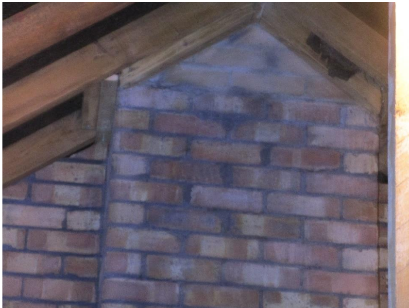
12 Interior – Roof Void – Party wall fully built up – staining to chimney – appears historic.
