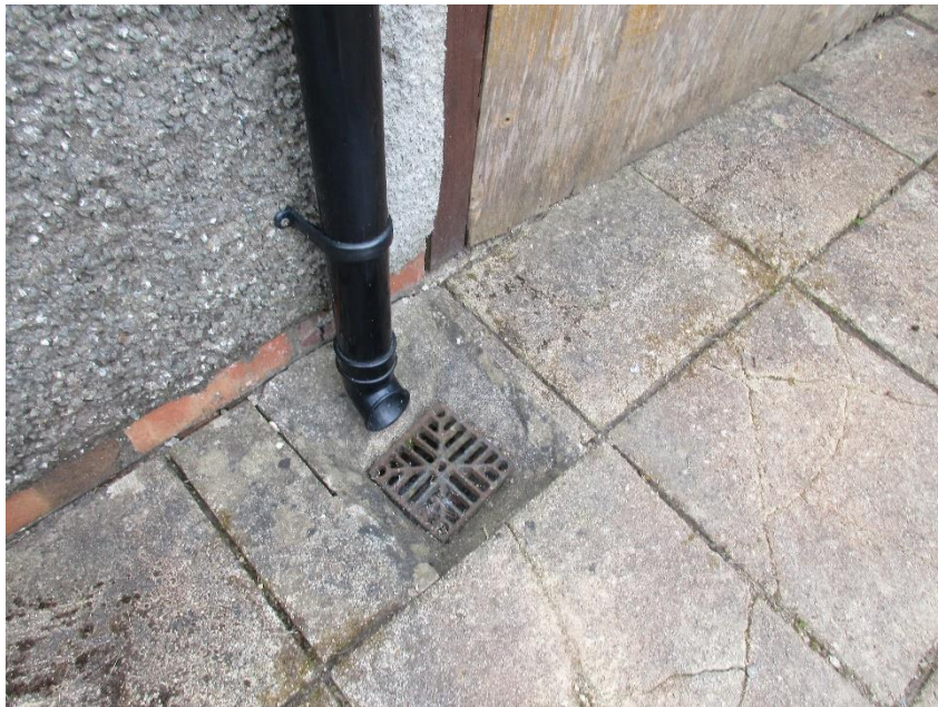
30 Exterior – Drains will require periodic clearing.
